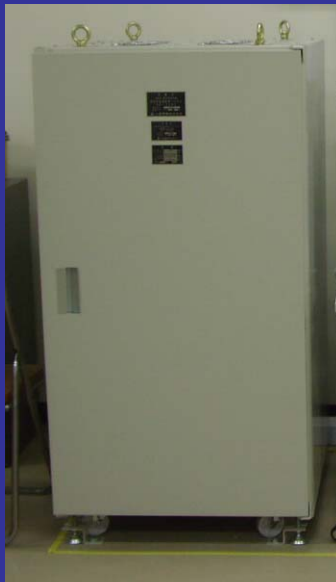
Transmitter and Receiver System
